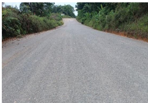
Fig. 4. Road conditions using Split+Basecourse.
